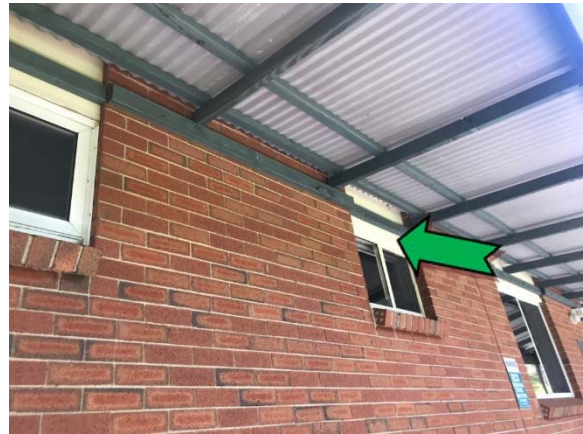
Photo 4. Exterior, throughout, high level infill panels above windows – assumed non asbestos-containing fibre cement sheeting.
