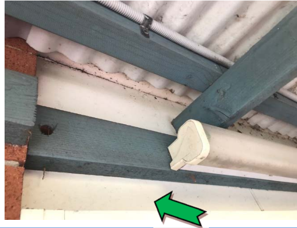
Photo 2. Exterior, north-east elevation, high level infill panels above window – non asbestos-containing fibre cement sheeting.
