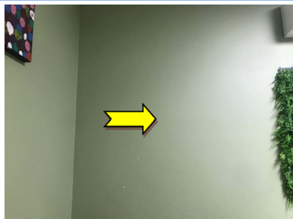
Photo 18. Interior, throughout, walls – suspected lead-containing dark green upper paint system
