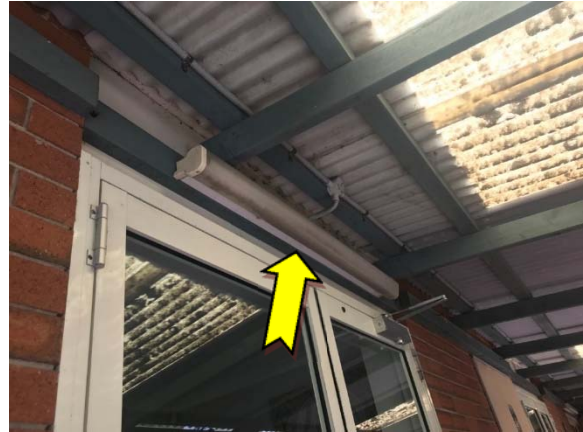
Photo 14. Exterior, throughout, single tube fluorescent light fitting – suspected PCB containing capacitor.
