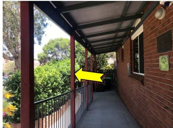
Photo 16. Exterior, throughout, verandah, timber beams – suspected lead-containing red upper paint system.
