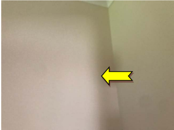
Photo 19. Interior, toilet 1, throughout, walls – suspected lead-containing light yellow upper paint system.
